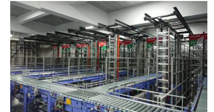
Automated case storage
